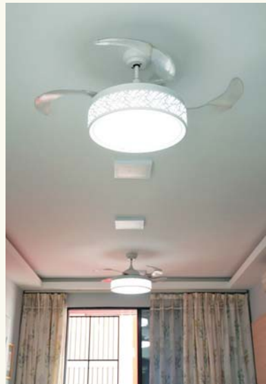
Eng bought all the LED ceiling fans in their home online.
